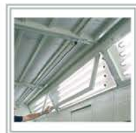
Eight 4-Tube LED light fixtures with hinged access for ease of cleaning and maintenance.
